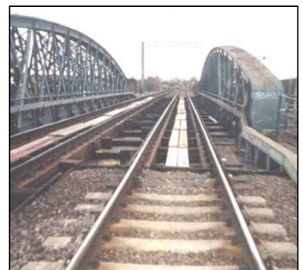
The track on the bridge cannot be lifted with jacks.
