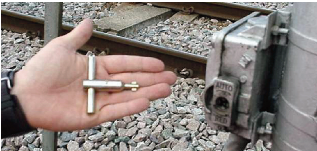
Signal-post replacement key and switch
