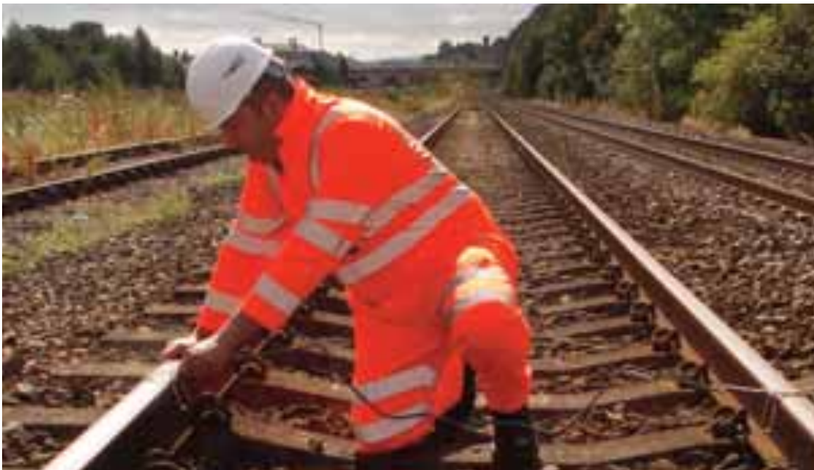
Using a track-circuit operating clip
