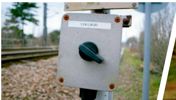
Example of a TOWS switch
