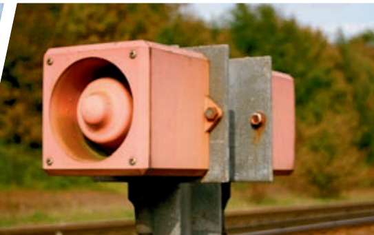
Example of a TOWS warning siren
