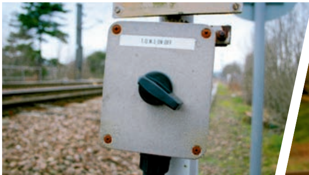
Example of a TOWS switch
