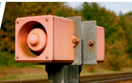
Example of a TOWS warning siren
